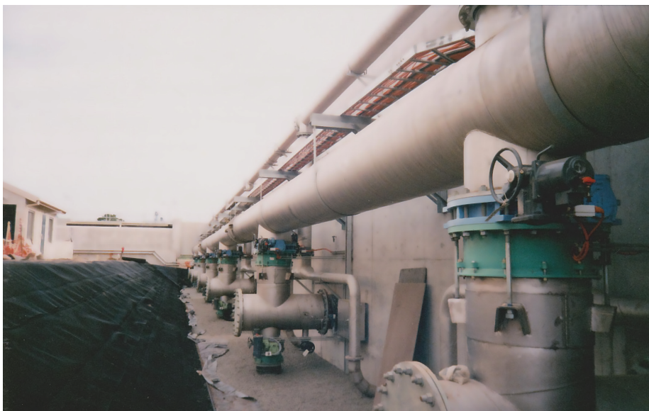
Appin Sewerage Treatment Plant, NSW. Fabricated and installed by ASSDA member and Accredited Fabricator Roladuct Spiral Tubing Pty Ltd using 316 grade stainless steel. Image courtesy of Roladuct Spiral Tubing Pty Ltd.
