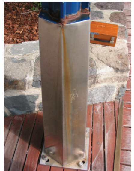
FIGURE 4: Example of a carbon to stainless steel weld with an inadequate coating
