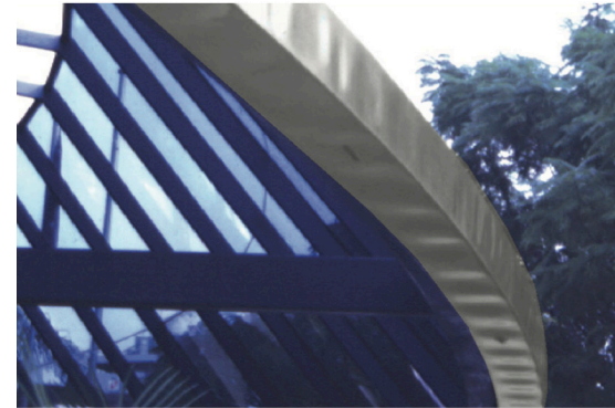
Ripples caused by welding practice.
