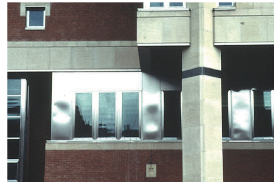
Buckling caused by insufficient allowance for solar heating.
