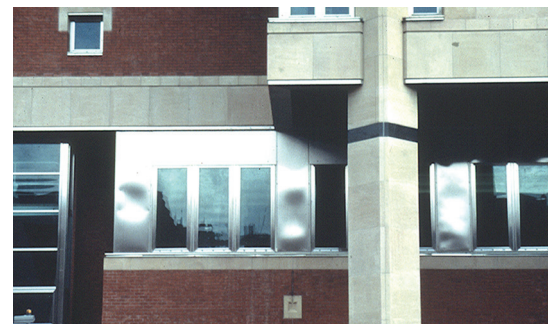
Buckling caused by insufficient allowance for solar heating.
