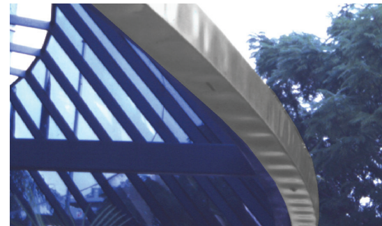
Ripples caused by welding practice.
