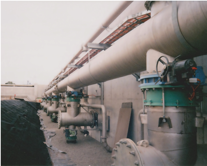
Appin Sewerage Treatment Plant, NSW. Fabricated and installed by ASSDA Member and Accredited Fabricator Roladuct SpiralTubing using 316 stainless steel.
