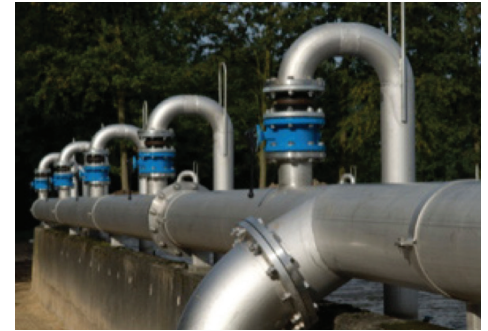
316 header in water treatment plant.
