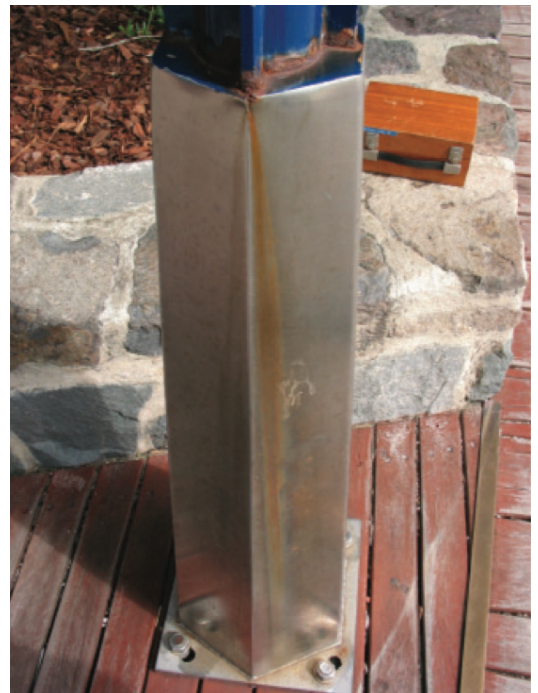
FIGURE 4: Example of a carbon to stainless steel weld with an inadequate coating
